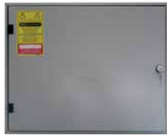
Machine room door
